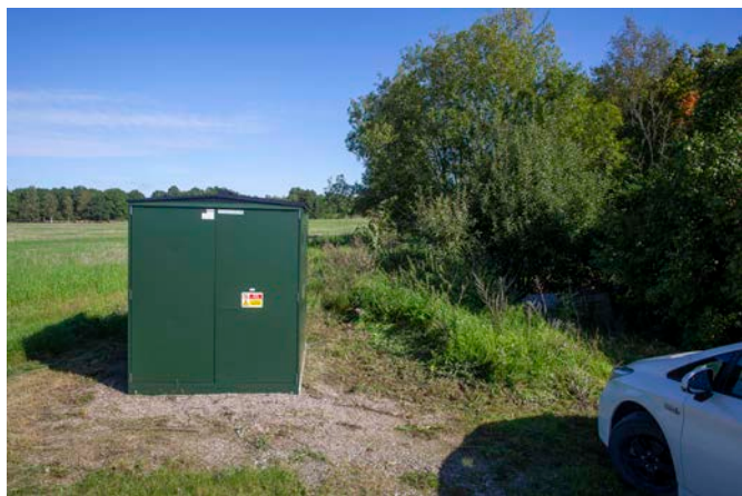
1. Transformatorstation innan Sandåker
