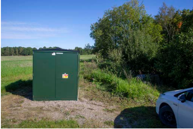
1. Transformatorstation innan Sandåker
